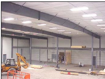
Bergstrom’s Service Department provided 800 amp service and lighting to this farm shop near Fisher, MN.
